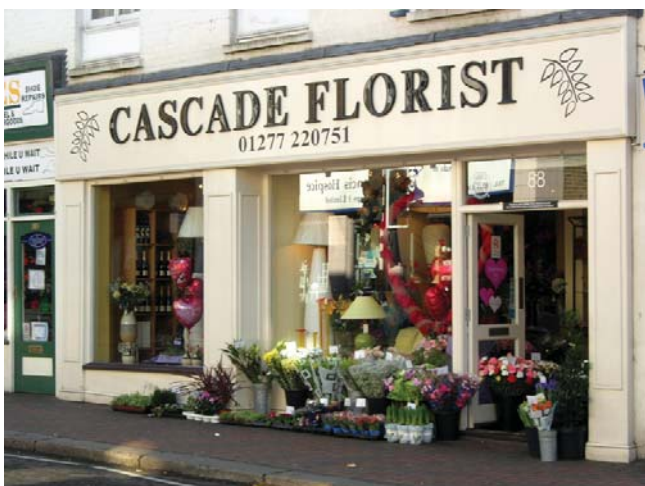
Cascade Florist: Generally a good example of a shopfront and one of the best along the High Street. Points to still consider include the size of the fascia- it is too deep. This may be a consequence of a reduced ceiling height in the ground floor shop. There are ways of reducing the fascia without disturbing the internal ceiling height. Street displays add interest and colour to the High Street but they need to be carefully controlled and considerate to all High Street users.
